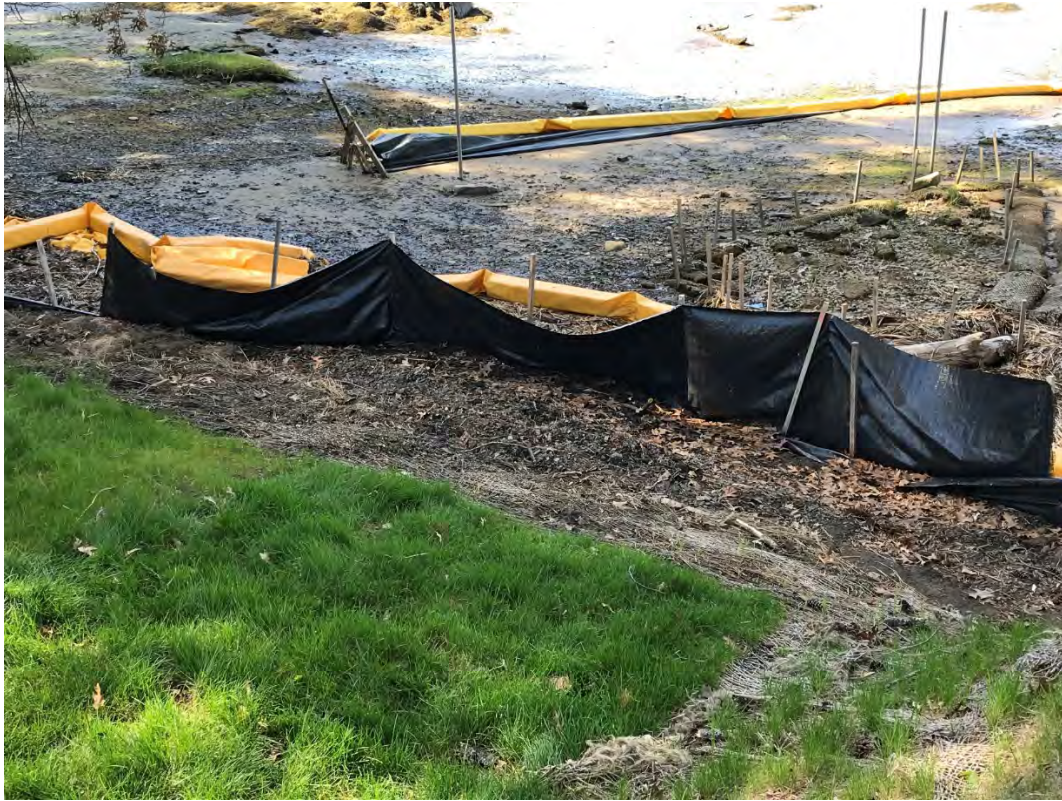
Fig 11: Toe of the slope at Gundalow Landing/east side of the bay. Viewing south. (05-11-21)
