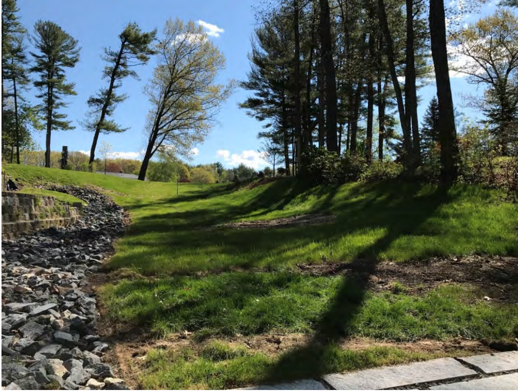
Fig 9: Slope above the manhole at Gundalow Landing/east side of the bay. Viewing east. (05-11-21)
